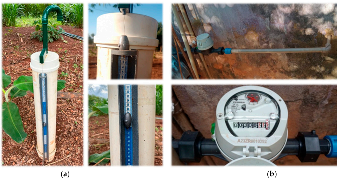
Figure 3. Level measurement mechanism (a) and water meter installed before the toilet bowl to measure the volume of water used for flushing (b).
