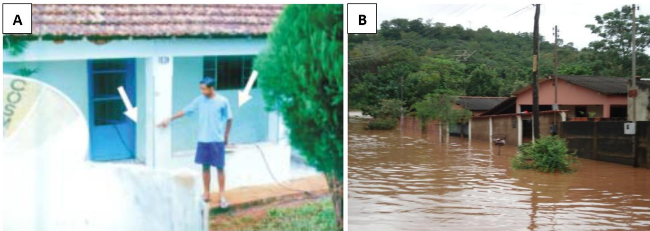
Figure 3: A) House showing signs of flooding in 2002. Source: SCOPEL et al. (2002). B) Flood in 2010. Source: Jatainews (2010).
