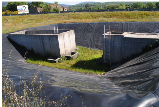
Figure 1: Detention basin for road runoff.
